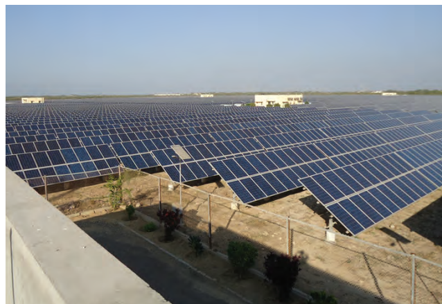
TPREL solar panel installations
