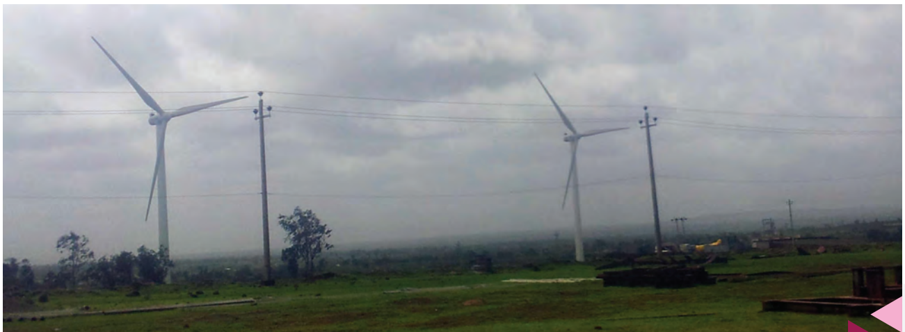
Windmill installed at Doddanavar Global Energy
