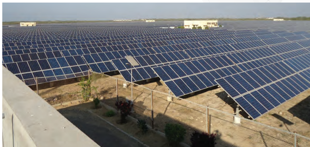
TPREL Solar Panel Installations
