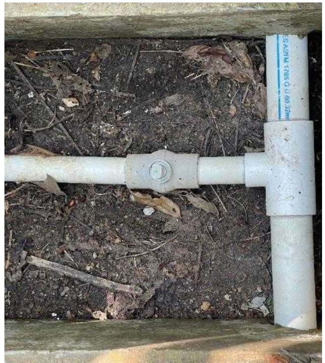
Figure 13: Water systems connection at Miyawaki site in Jewel Garden
